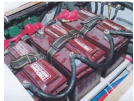
The Tartan has a robust electrical system, with a standard pair of group 27 Trojan deep cycle batteries (plus a third on the test boat).
